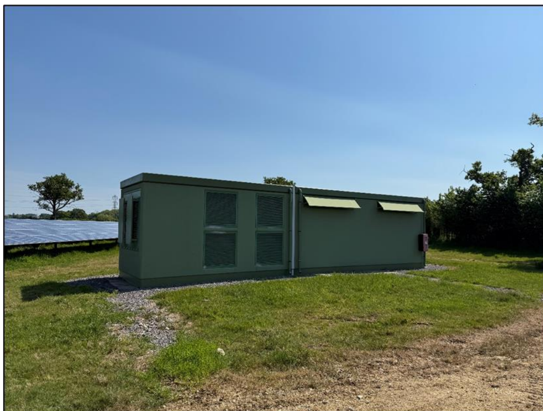
Plate 2-8 Typical 33kV Switch room
